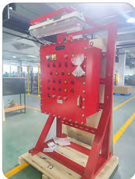
8. Application of explosion-proof control system for fire pumps
